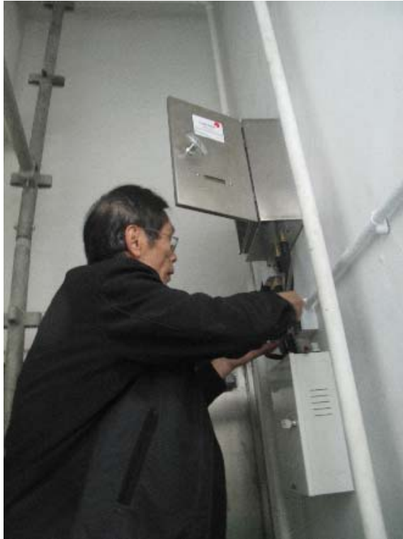
Installation of MPS Control Units
